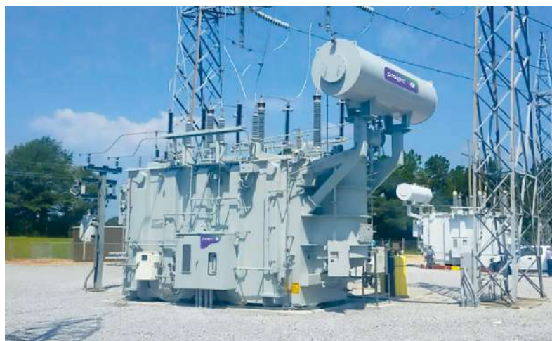
World's First Large Flexible Transformer
